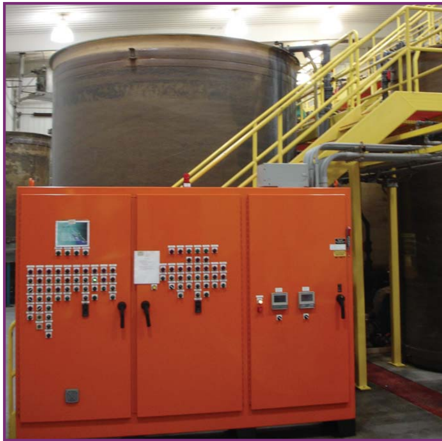
Professional Plating made a $1.5 million wastewater expansion in 2001—years ahead of the rush toward more stringent compliance measures.
